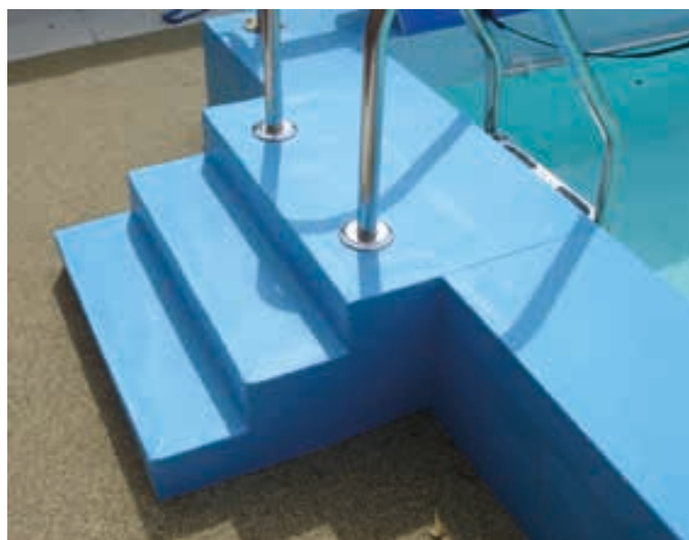
Photograph supplied by Hutchings and Carter
