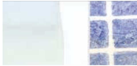
Liners that have come in contact with sun cream and chlorinated water.
